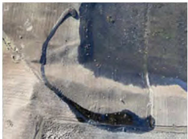
Water was found under some of the repairs, these have also failed
