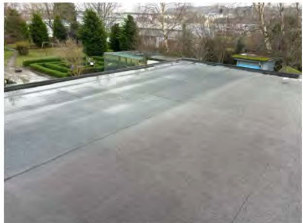
Different mineral cap sheets noted in the picture above shows a historic repair
