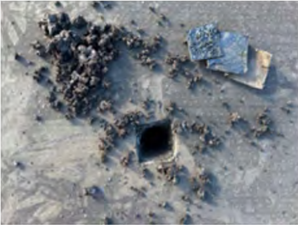
Core on lower roof shows cork saturated
