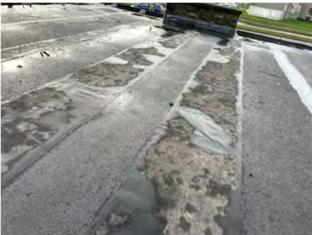
Repairs were noted on both the main and lower roofs to have historically been carried out with many different materials
