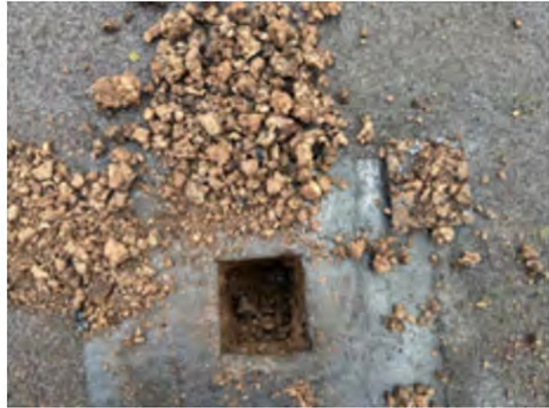
Cork on the main roof was dryer though has debonded in places from the cap sheet
