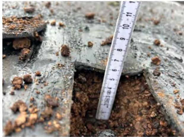
Cork in low point of the roof shows cork is 40mm deep
