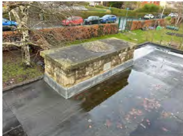
Additional ponding just outside the gutters was also noted
