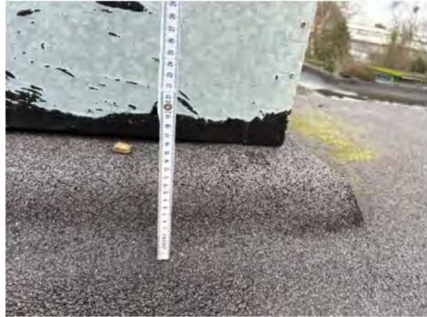
Vent kerb will require to be raised to meet BS6229
