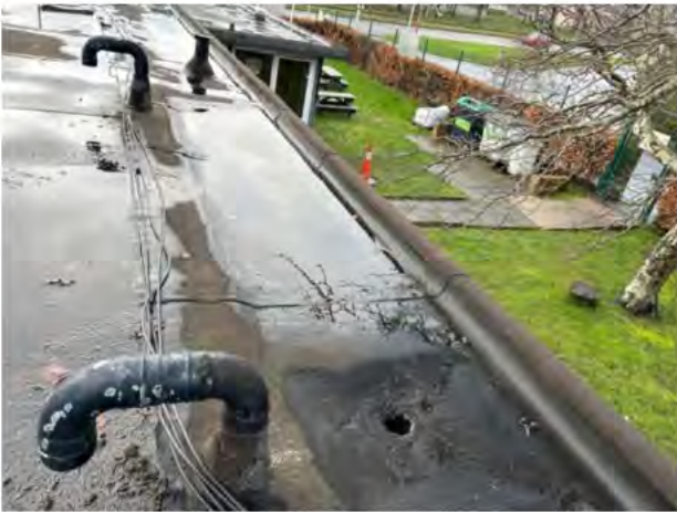
Confirmation if the downpipes are still in use and what their task is
