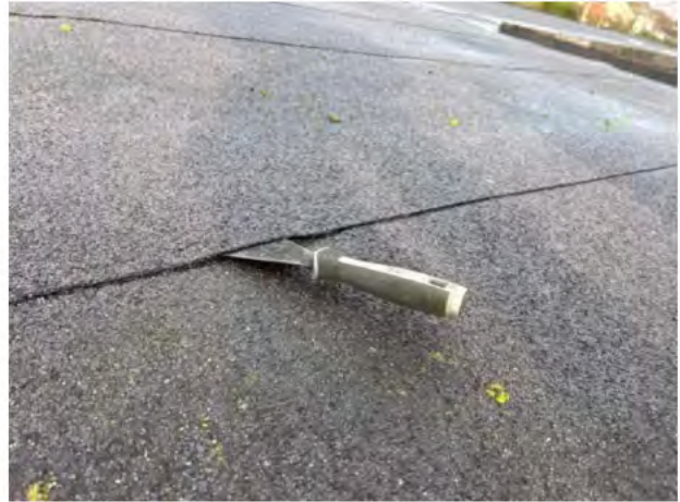
Loose laps were found over the roof area
