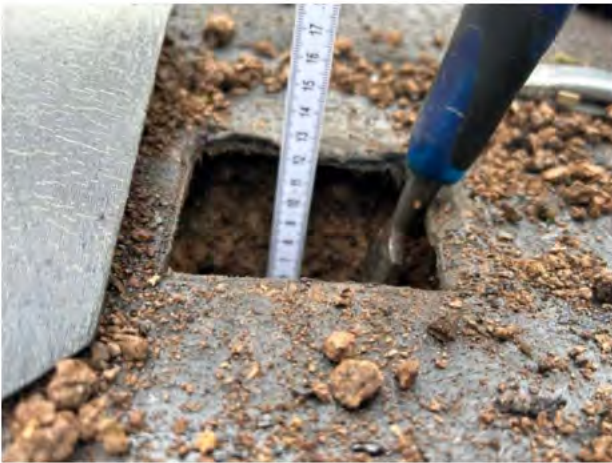
Core in high point of the roof shows cork is 110mm deep
