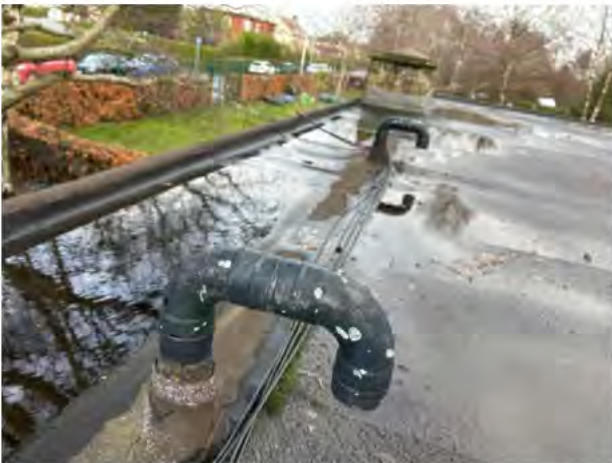
Ponding in the gutters was evident on inspection
