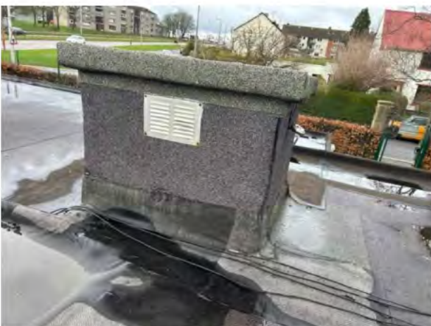
Bare faced felt repairs were also evident to have been carried out on the roof areas
