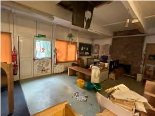
Partial ceiling collapse internally and water ingress shows the existing waterproofing system and drainage has failed
