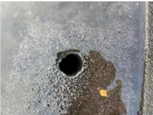
The current outlets are very narrow and poorly detailed
